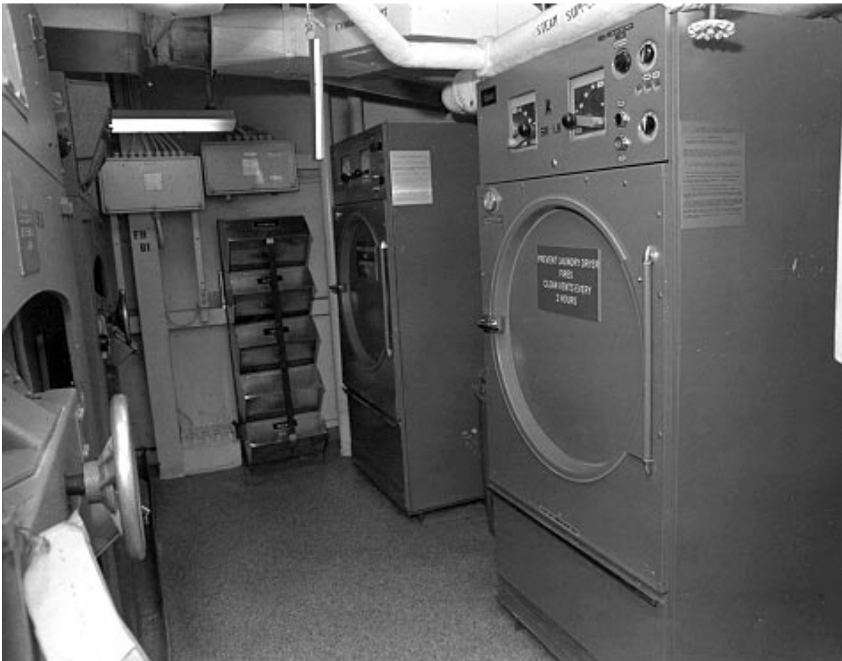
Figure 5-23.-Battery of tumble dryers.
